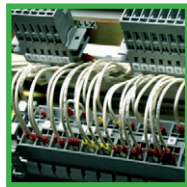
Electrical cabinets and substations
